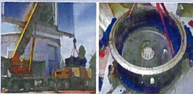
The first of the telescope pieces to go in was the pedestal, shown above being lifted out of its crate (left) and being placed on the bolt pattern (right). Most of the large pieces are being hoisted by crane through the open shutter doors of the dome, and are then lowered into place.
