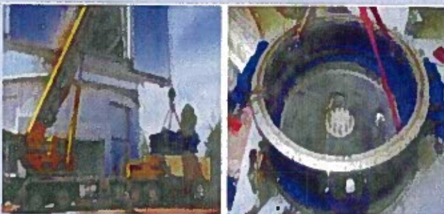
The first of the telescope pieces to go in was the pedestal, shown above being lifted out of its crate (left) and being placed on the bolt pattern (right). Most of the large pieces are being hoisted by crane through the open shutter doors of the dome, and are then lowered into place.
